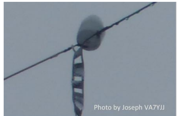
Ice formed between uninsulated poles of dipole
